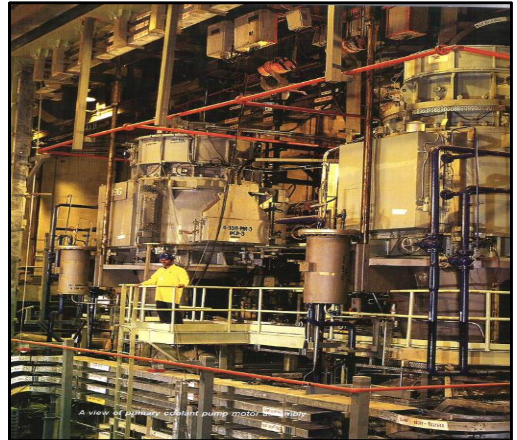
Reactor Coolant Pump
